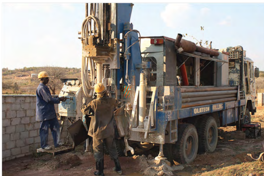
Construction of water Borhole at Ubaru-Igbariam Community in Anambra East LGA of Anambra State (EU-UNICEF Water Supply and Sanitation Sector Reform Programme-II (WSSSRP-2PHASE-3 lot 26)
