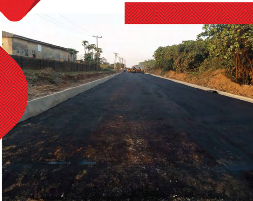
Construction of Internal Roads of Ikot Ekpene Medium Prisons [drainages], Akwa Ibom State.
